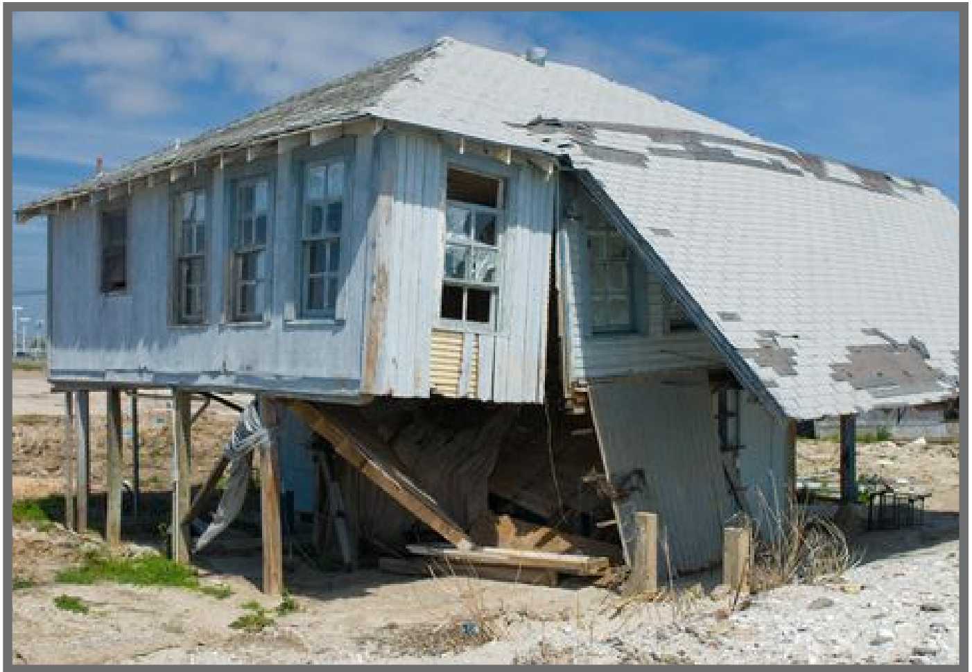
Aftermath of Hurricane Katrina
